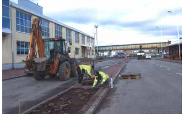
In 2008, street and field areas were elevated in the passenger harbour area and the boundary wall of the Kanavaniemi quay was heightened due to increasingly common flooding. The tiling and elevation work in Ensimmäinen linja street commenced in April 2008 and the work for flood prevention was completed in June 2008.
